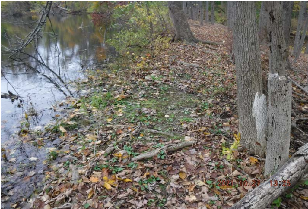
Photo 3 Dam ID# 195-1592 Sky View Pond Dam 10/27/2021 Low spot on dam crest towards right end (almost no freeboard) View looking right
