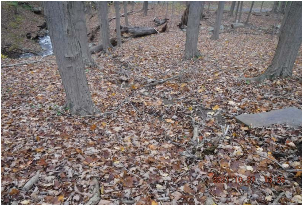
Photo 5 Dam ID# 195-1592 Sky View Pond Dam 10/27/2021 Evidence of overflow on downstream slope towards the spillway View looking downstream from crest
