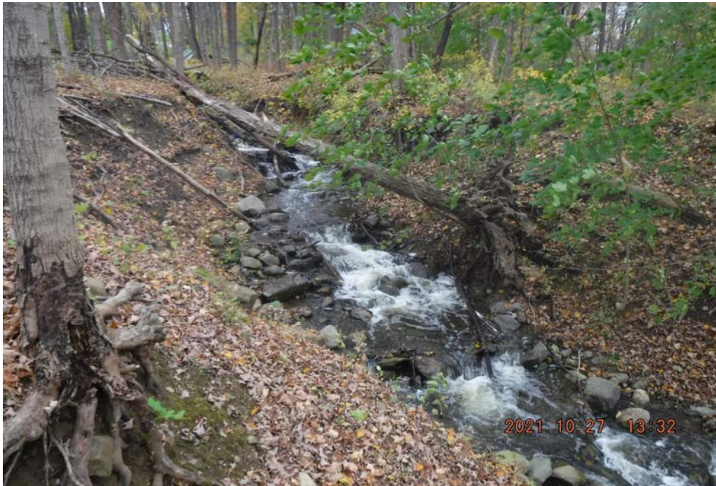
Photo 13 Dam ID# 195-1592 Sky View Pond Dam 10/27/2021 Service spillway downstream outlet channel View looking upstream from outlet channel Note: visible signs of embankment erosion in downstream channel
