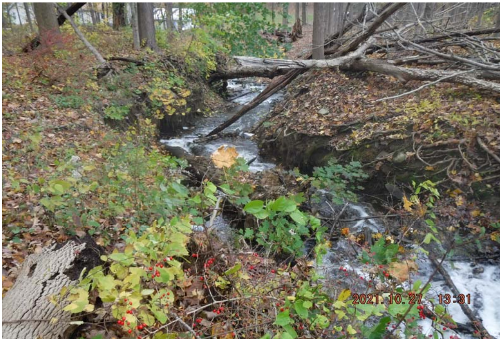
Photo 12 Dam ID# 195-1592 Sky View Pond Dam 10/27/2021 Service spillway downstream outlet channel View looking downstream from service spillway Note: visible signs of embankment erosion in downstream channel
