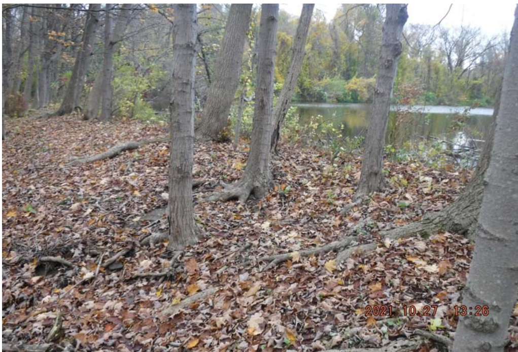
Photo 4 Dam ID# 195-1592 Sky View Pond Dam 10/27/2021 Evidence of overflow on downstream slope towards spillway View looking right from left side
